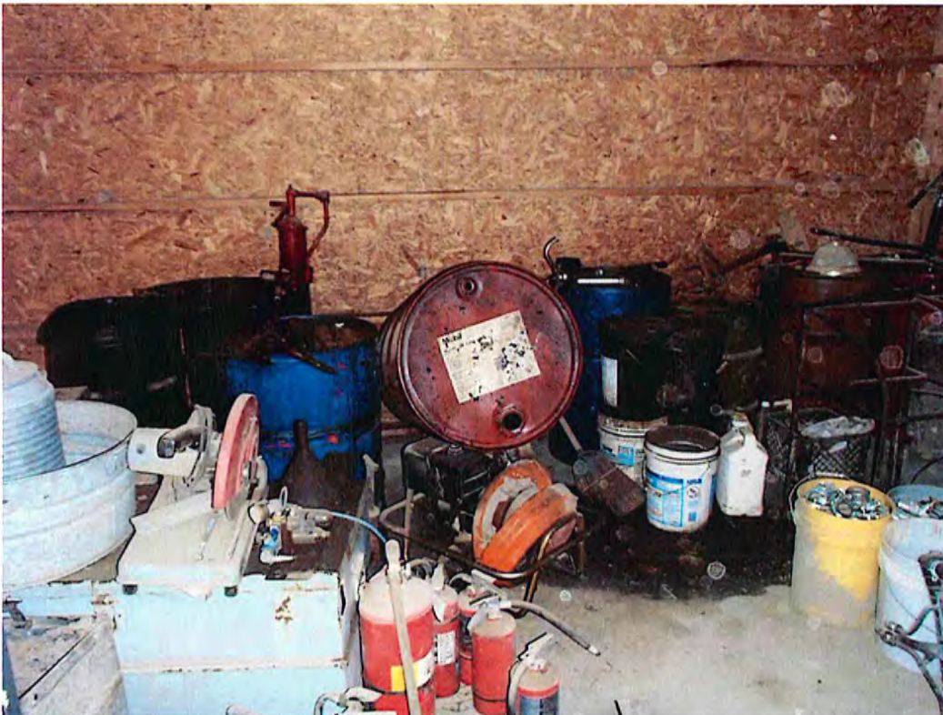
Date: 10/16/2013 Time: 1:22 P.M. Direction: south Photo by: Garrison Gross Exposure #: 010 Comments: used / waste automotive fluids; drums not labeled; fluids spilled on floor
